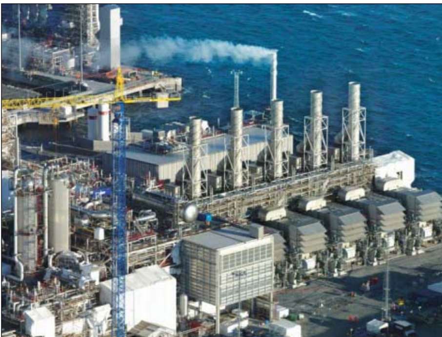
Five LM6000 gas turbines provide power for the plant, with the backup of the regional grid. Instead of direct mechanical drive, however, the refrigerating compressors are driven by electric motors (Fig. 5; photo by Harald Pettersen, Statoil).
